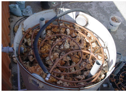
Fig. 3.4: Biofilter 1 with sand and gravel layers
